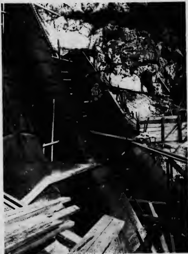
Coquitlam-Buntzen Development. Pipe Lines Nos. 1, 2 and 3, Plant No. 2, Lake Buntzen.
